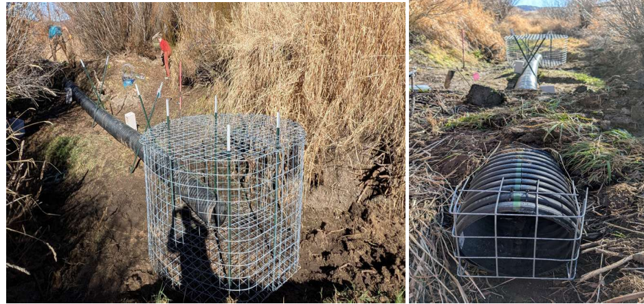
Figure B-19. Pond leveler installed in an intermittent stream to prevent flooding on private property in Routt County. Photos provided by Emily Burke and Ryan Messinger.
