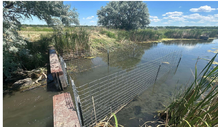
Figure B-7. Exclusion fencing installed by Nick Hagan (Songdog Outdoor Services/BeaverCorps Member) in a spring fed slough to protect a check gate from beaver clogging it up that CPW uses to raise and lower water level for waterfowl habitat at the Elliott State Wildlife Area along the South Platte River, near Brush, CO. To avoid a channel-spanning fence on the upstream end, this design lacks the typical outward "flare" seen in most trapezoidal/Keystone fences. Photo by Nick Hagan.
