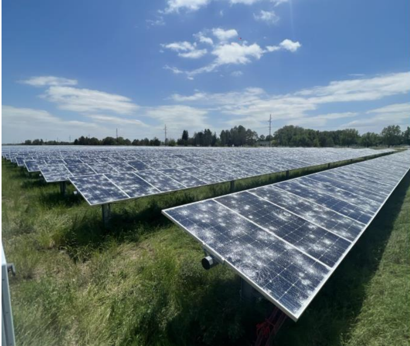
Figure 3: Field of destroyed solar panels after a hailstorm; not so resilient after-all.
