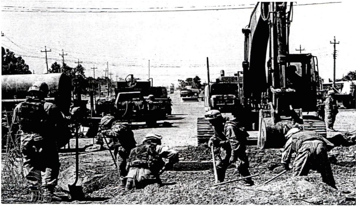
In Fallujah, Seabees worked to prepare the site for the construction of a bridge in 2006.
