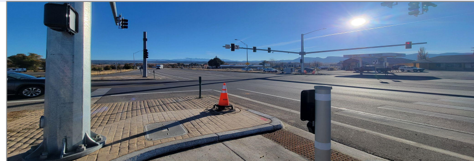
Region 5 - Cortez Public Right-of-Way Accessibility Guidelines (PROWAG)/Americans with Disabilities Act (ADA) Signal and Ped Pole upgrades
