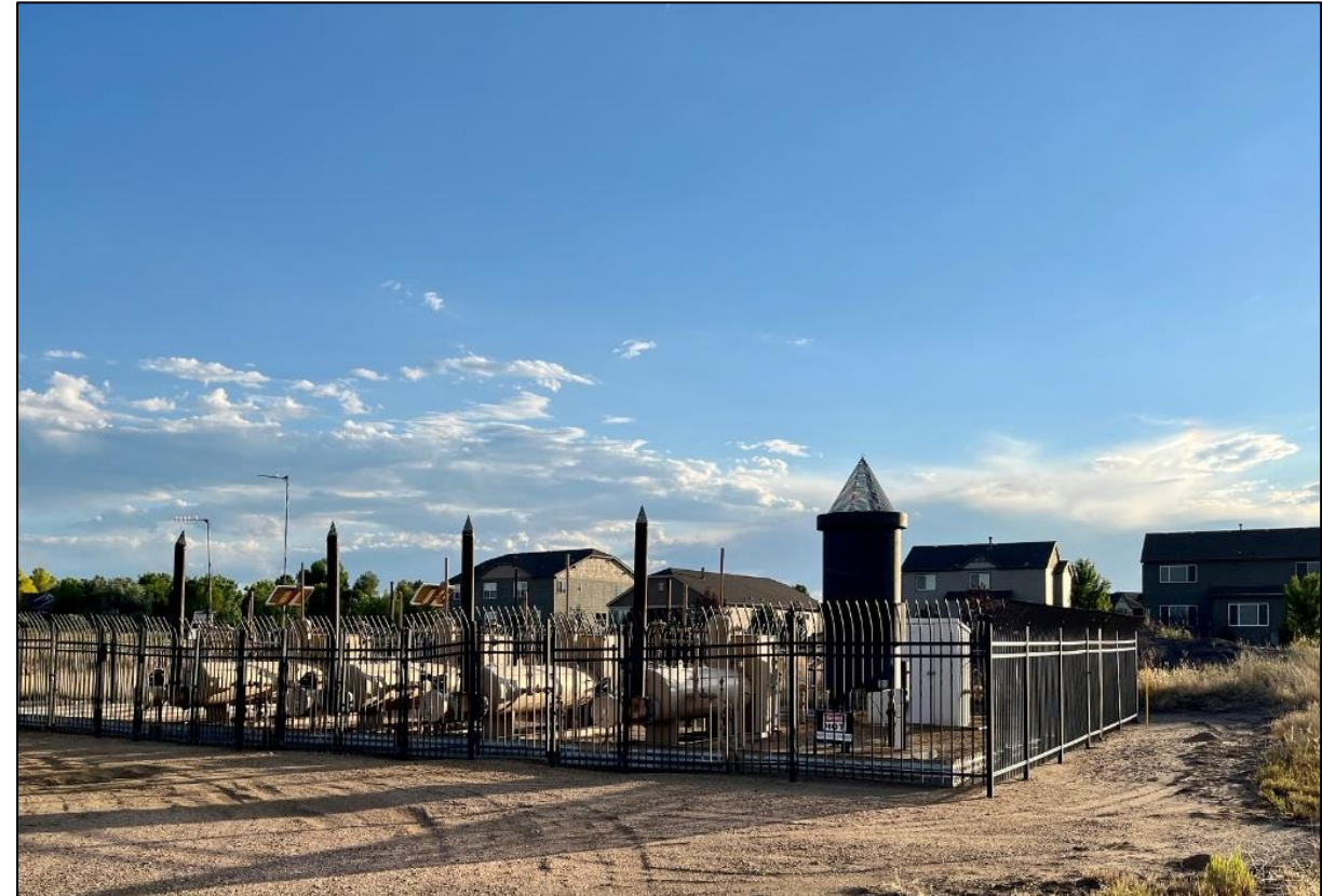
Oil and gas infrastructure in Boulder County
