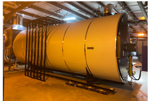
ACRE 3 funding helped replace two 9-megawatt boilers at BrushCo, a greenhouse in Brush.
