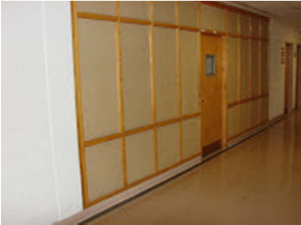
Building A: Hallway glass wall replaced by plywood
