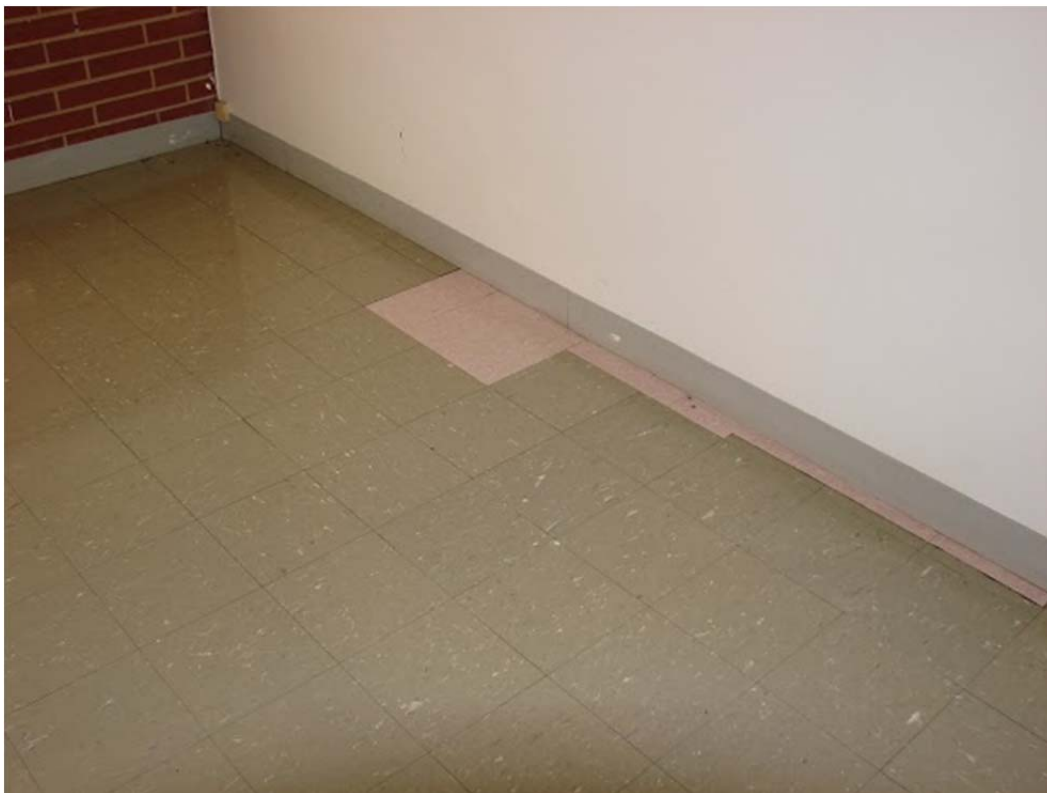
Building KC: Asbestos floor tiles
