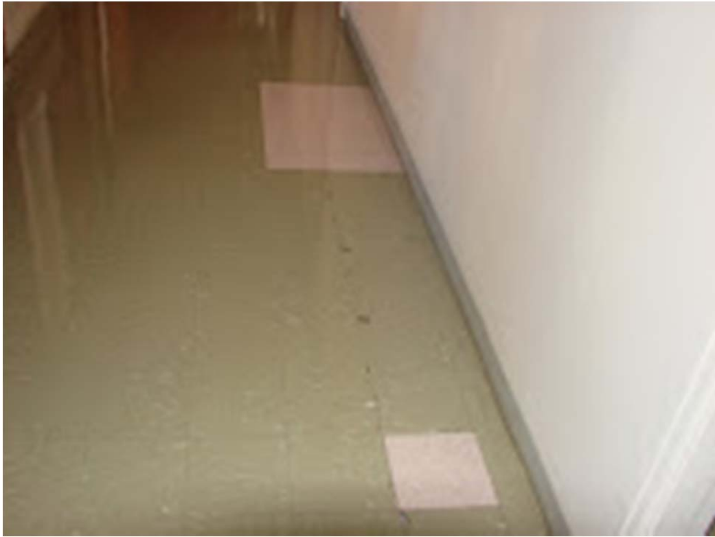
Building KC: Surface mold on the floor
