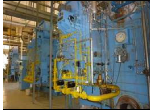
Figure 17: Parcel D – Boiler Plant Interior
