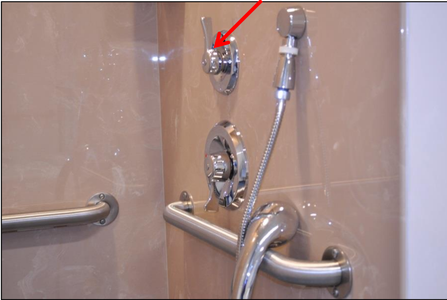
Photo A: Shower/Bath fixture
