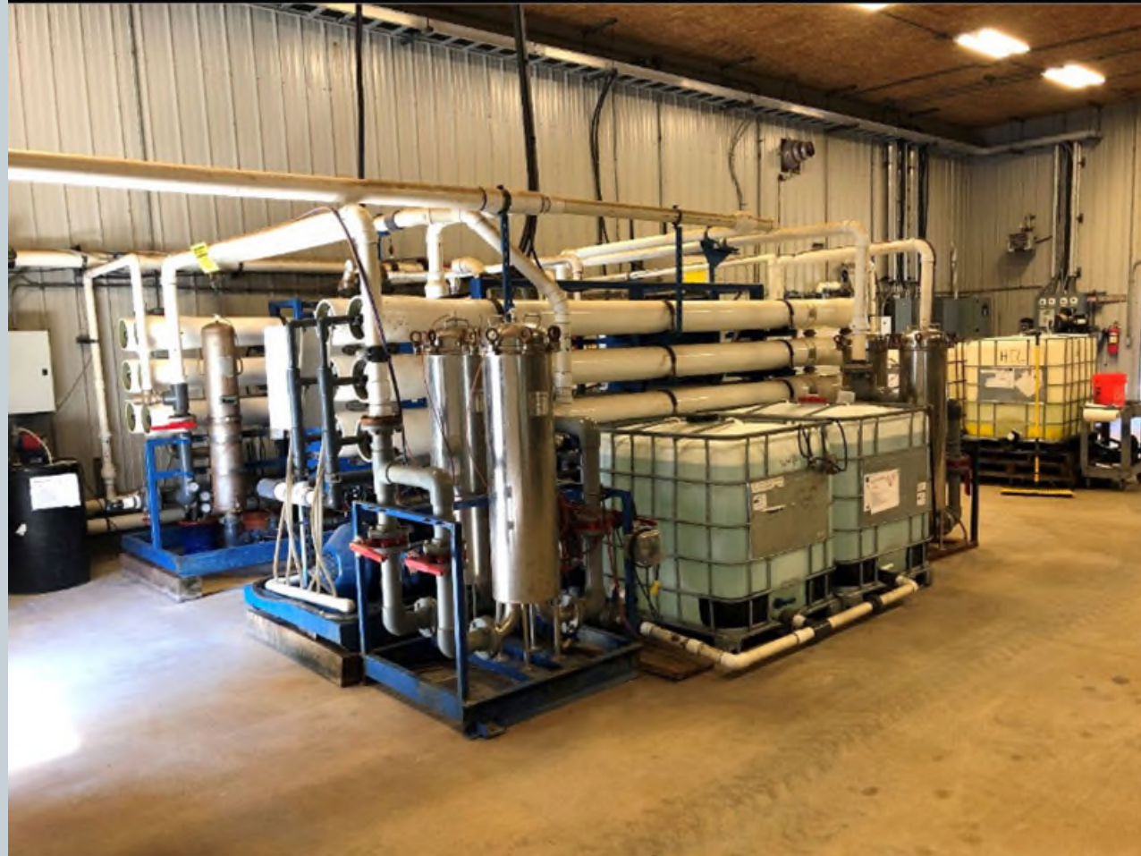
Reverse Osmosis System
